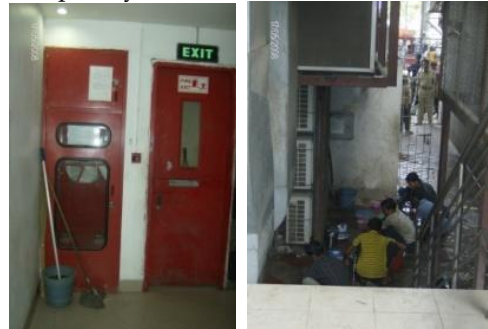
Figure 10: Closed Fire exit and its out side
