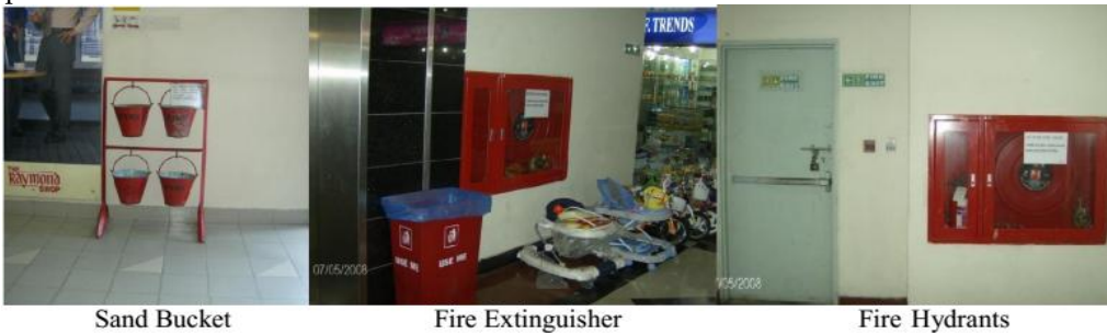
Figure 13: Fire Fighting Equipments
